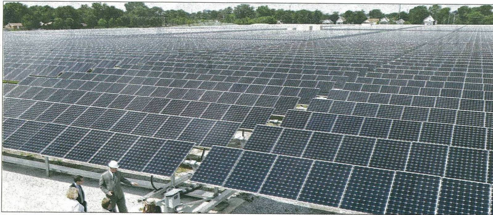
Exelon has completed its $60 million solar panel project that began operation in December at 1201 W. 120th St. in West Pullman. | JOHN J. KIM-SUN-TIMES
